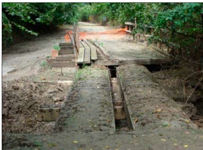
Flood waters moved this bridge from its foundation on the Steamboat Trace during the summer of 2010
