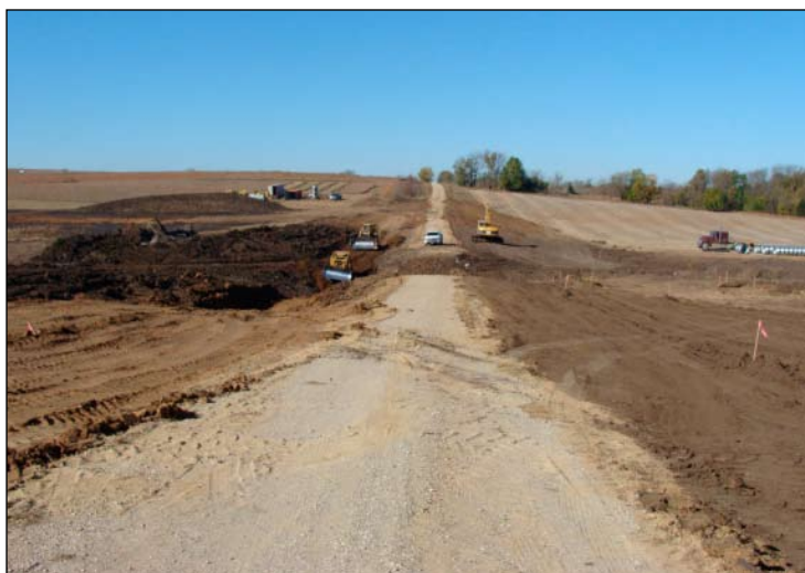
Don Bruna Construction works on the Ray Caspers road dam in October, 2010
