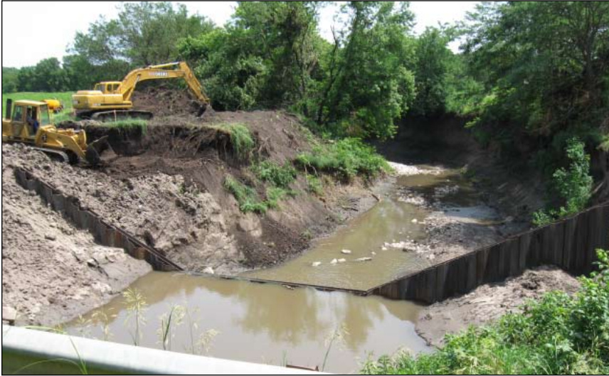
Work was completed this summer on this weir near Johnson in the Big Muddy Creek Watershed
