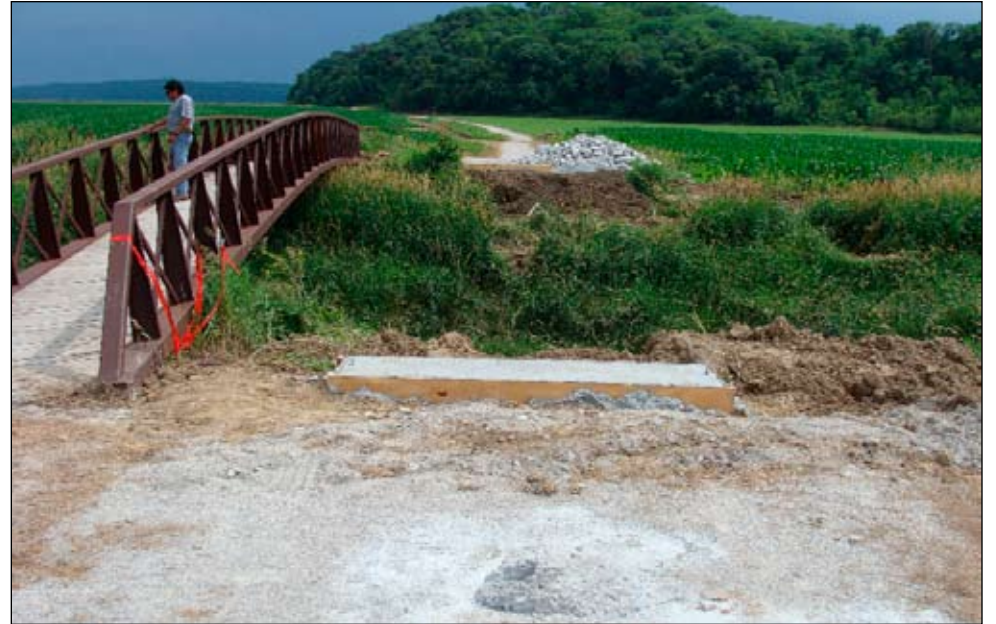
New concrete approaches were poured last summer to support this bridge across Honey Creek on the Steamboat Trace.
