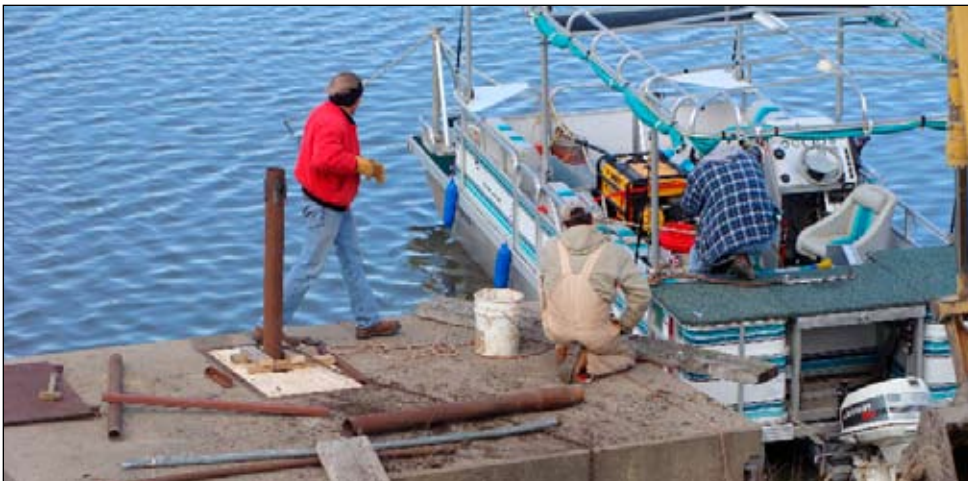
Crews work on replacing a defective drawdown valve at Iron Horse Trail Lake.
