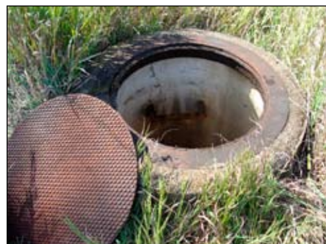
Abandoned wells like this one are scattered across the countryside in southeast Nebraska.
