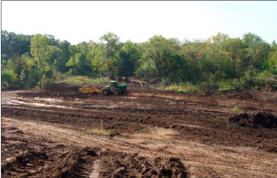
Muddy Creek Watershed dam under construction on Larry Bohlken property in September.
