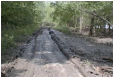
After waters receded a heavy layer of silt remained over many areas of the trail.
