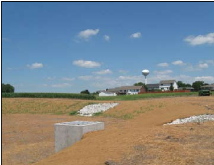
“This detention cell will temporarily hold future storm water before releasing it in a controlled manner.”
